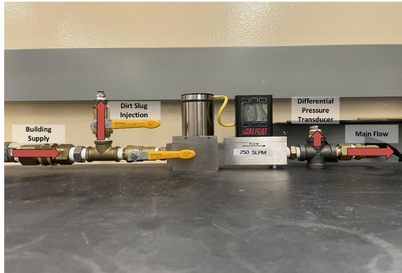
Figure 7. As-built flow control plumbing at U-M.
