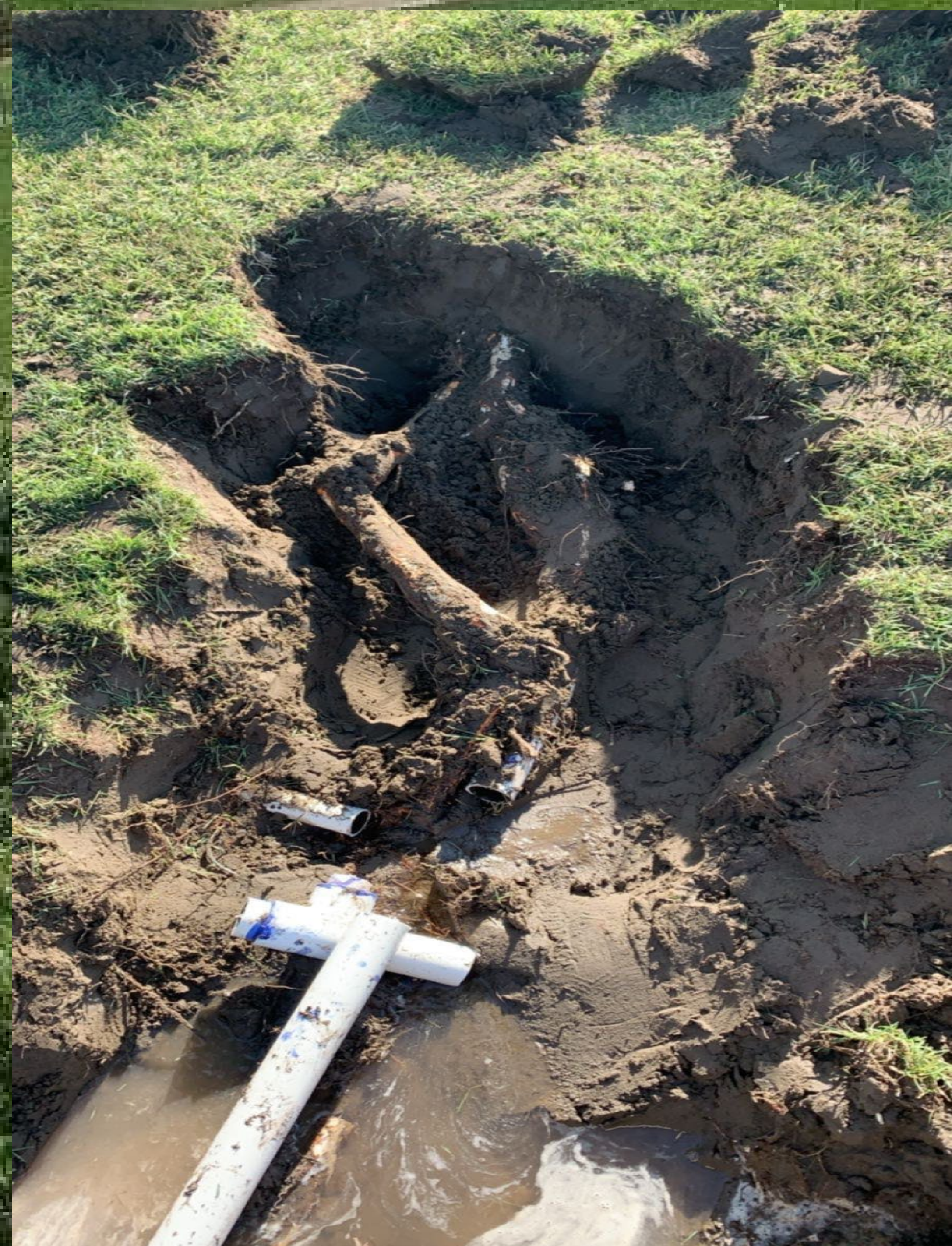
Figure 1: Broken pipe that had to be dug up and fixed, you can see tree roots that pushed into the pipe causing the breakage
