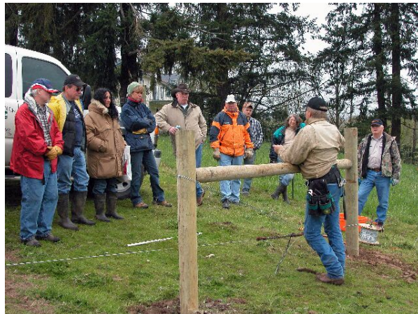
Gallagher Fencing staff demonstrate the installation of a cross brace in an electric fence.
