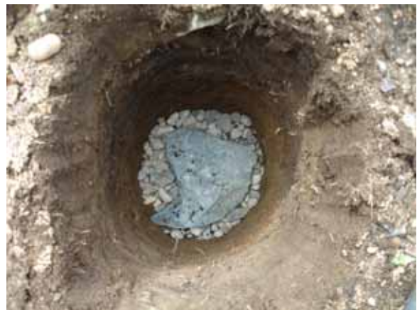
To plant your posts, dig a hole 2½ feet deep, add 6 inches of gravel, and place a chunk of flagstone on top of that to provide a sturdy base for your post.
