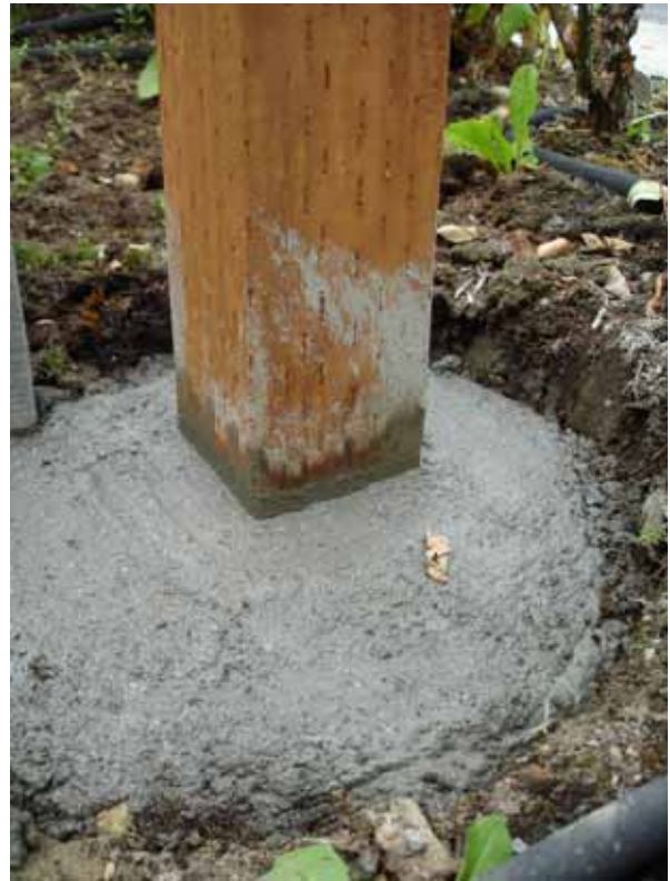
“Crown” the cement at the base of each fence post, shaping it so that it slopes away from the post. This will help move rain water away from the base of the post. Photo by Jason Miller
