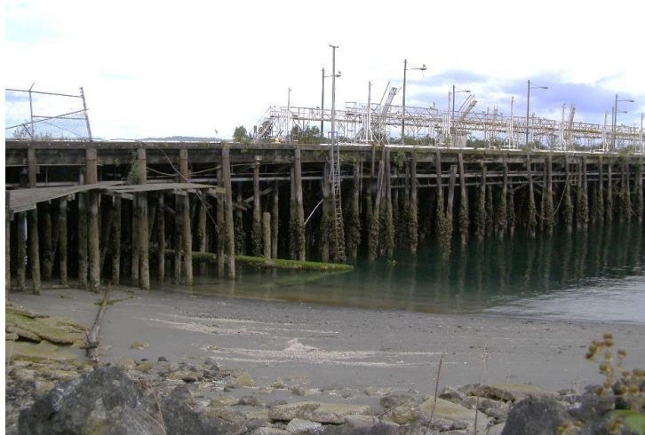
Creosote soaked timber piles at Mukilteo Tank Farm Pier (Photo: Washington DOT)
