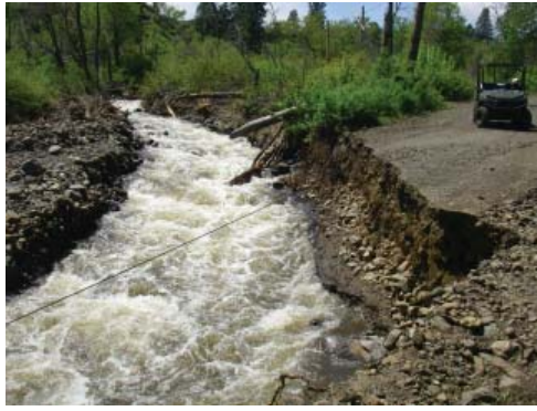
A flooded stream can find a new channel, cutting through roads. (Photo: Tip Hudson)
